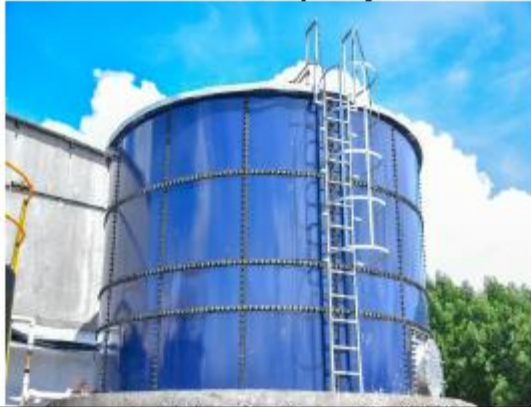
Intermediate Tanks Capacity: 15 KL
